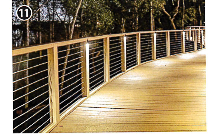
RAILING - WOOD RAILS AND POSTS AND S.S. CABLE WIRES
